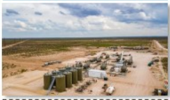
Separators, tank buffers, wellheads, etc.
