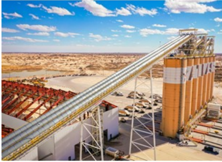
Atlas conveyor fed silos at Kermit Facility
